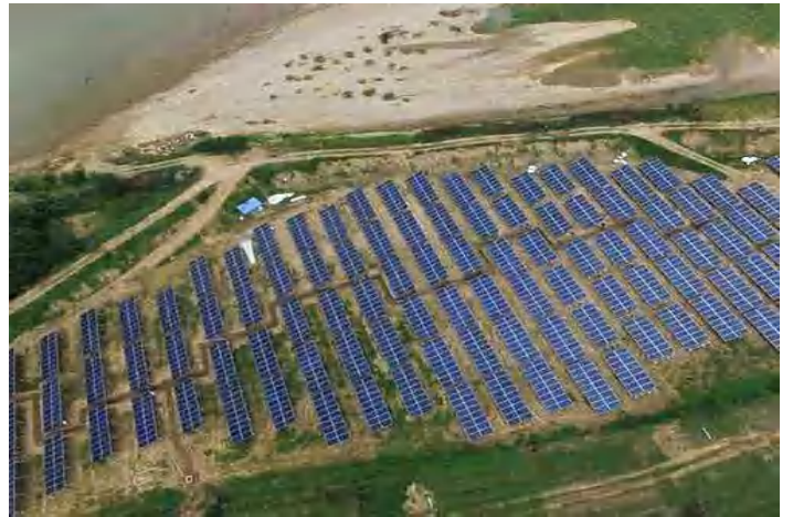
Location : Germany Capacity : 2MW
