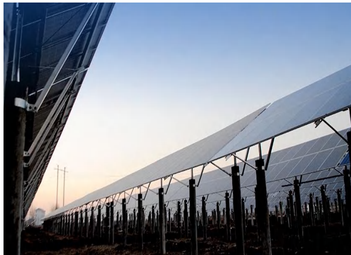
Location : Fuyang, China Capacity : 2MW
