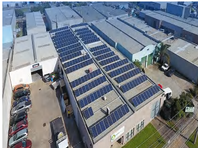
Location : USA Roof Top PV System Capacity : 70 KW
