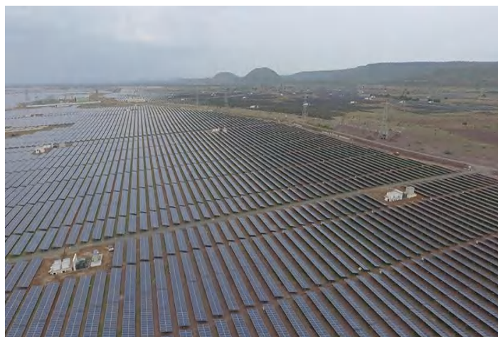
Location : Philippines Capacity : 5MW
